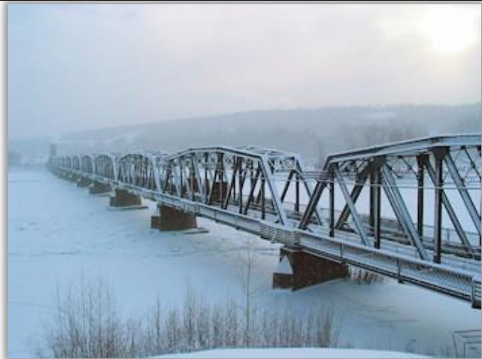
Railway Bridge, Prince George over the Nechako River Photos courtesy of UNBC Communications
